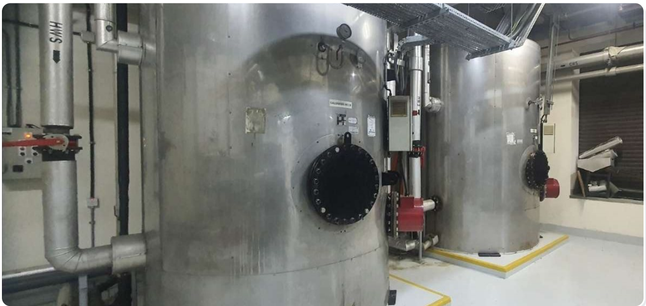
Hot & cold water tanks
